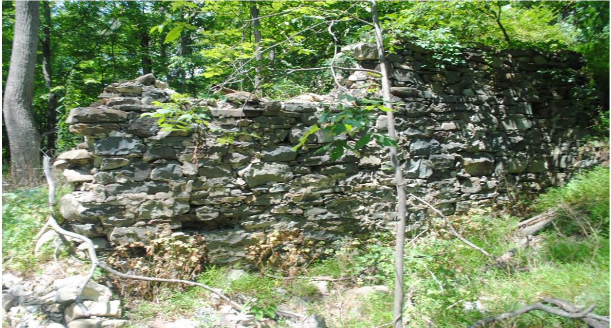
Photo 55: The various walls of the Howell foundation show several different construction styles. View to the north.
