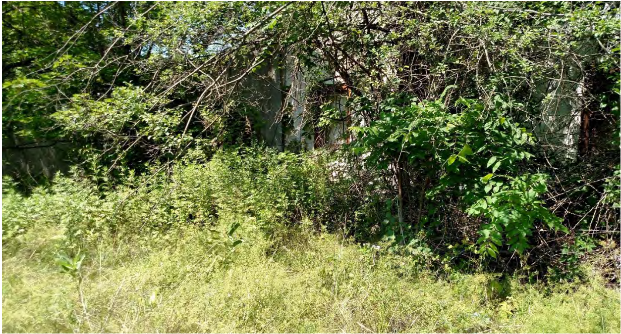
Photo 30: A wood frame addition connects the H. Howell house to the Quonset hut. View to the west. This elevation around the house is heavily overgrown with vegetation.
