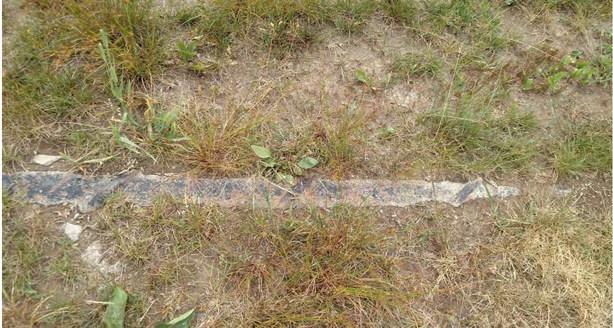
Photo 10: Area E contains subsurface iron infrastructure. View to the east.
