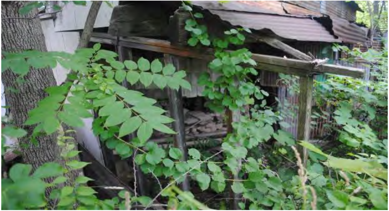
Photo 31: View of the dry laid field stone on the south western wall of the structure. The openings in the wall contain modern piping and have been reinforced with corrugated steel sheeting.
