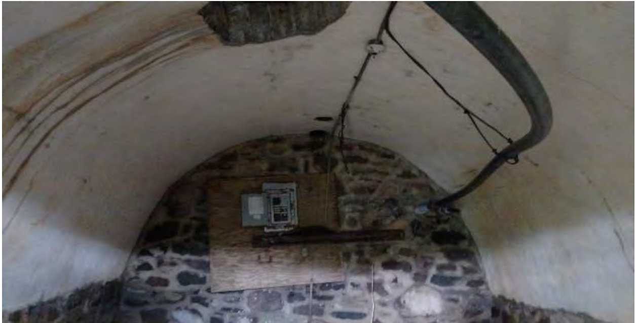
Photo 5: Interior of the spring house showing the modern electrical features.
