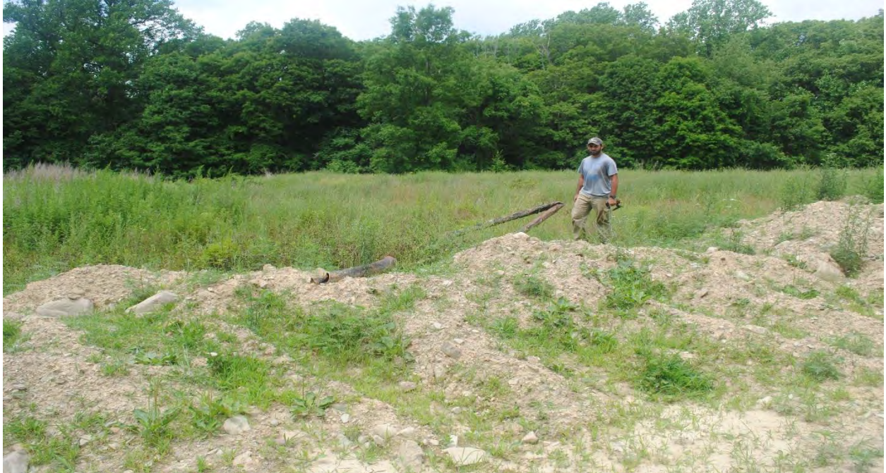
Photo 46: Within the former golf course earth moving activities had taken place to remove some of the former infrastructure. View to the north.
