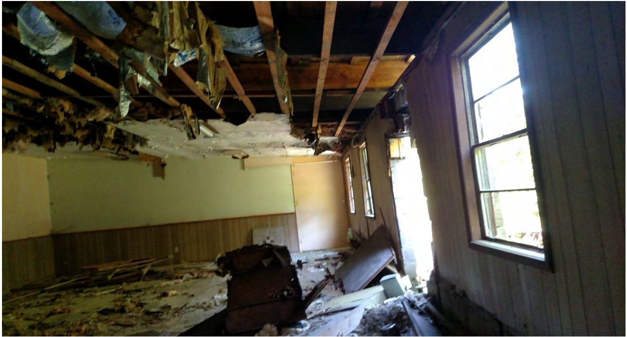
Photo 4: Interior of the Clubhouse structure. The exterior walls of the building along with the interior of the structure is degraded.
